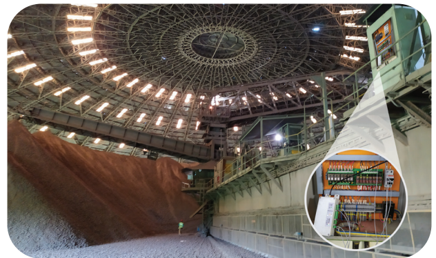
Circular Stacker Reclaimer Monitoring
